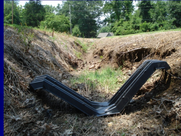
12" inadequate for portions
