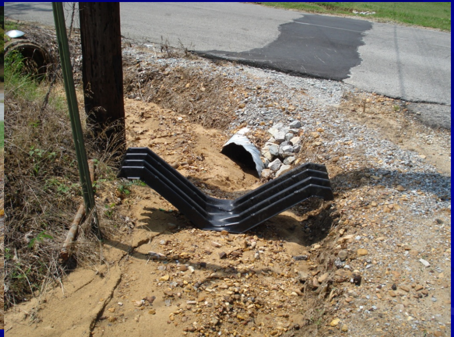
1' Ditch (deposition) on E. Main
