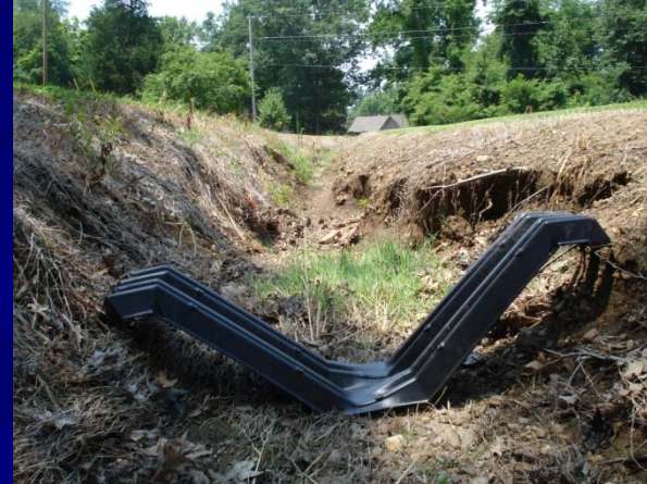
12" inadequate for portions
