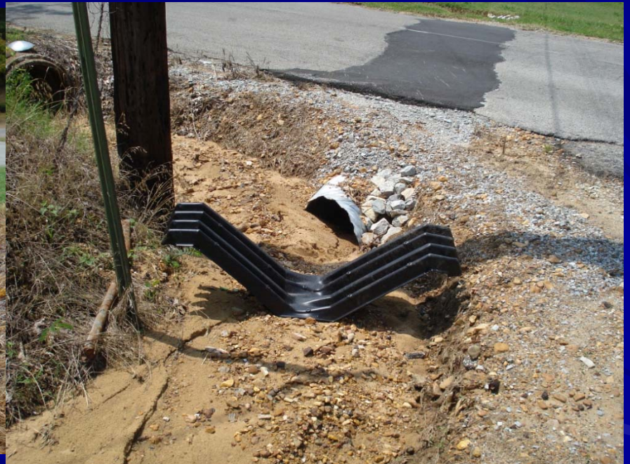
1' Ditch (deposition) on E. Main
